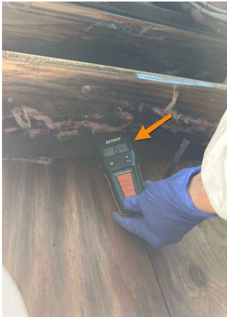
Moisture stained framing dry at 6% moisture
