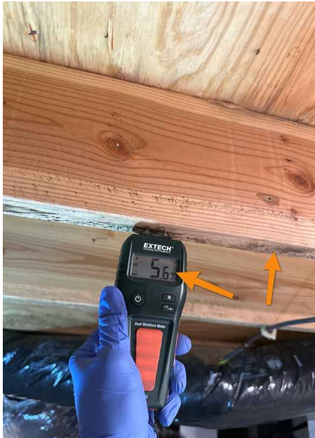
Surface fungus visible, inactive at 5% moisture, non-damaging type, considered cosmetic
